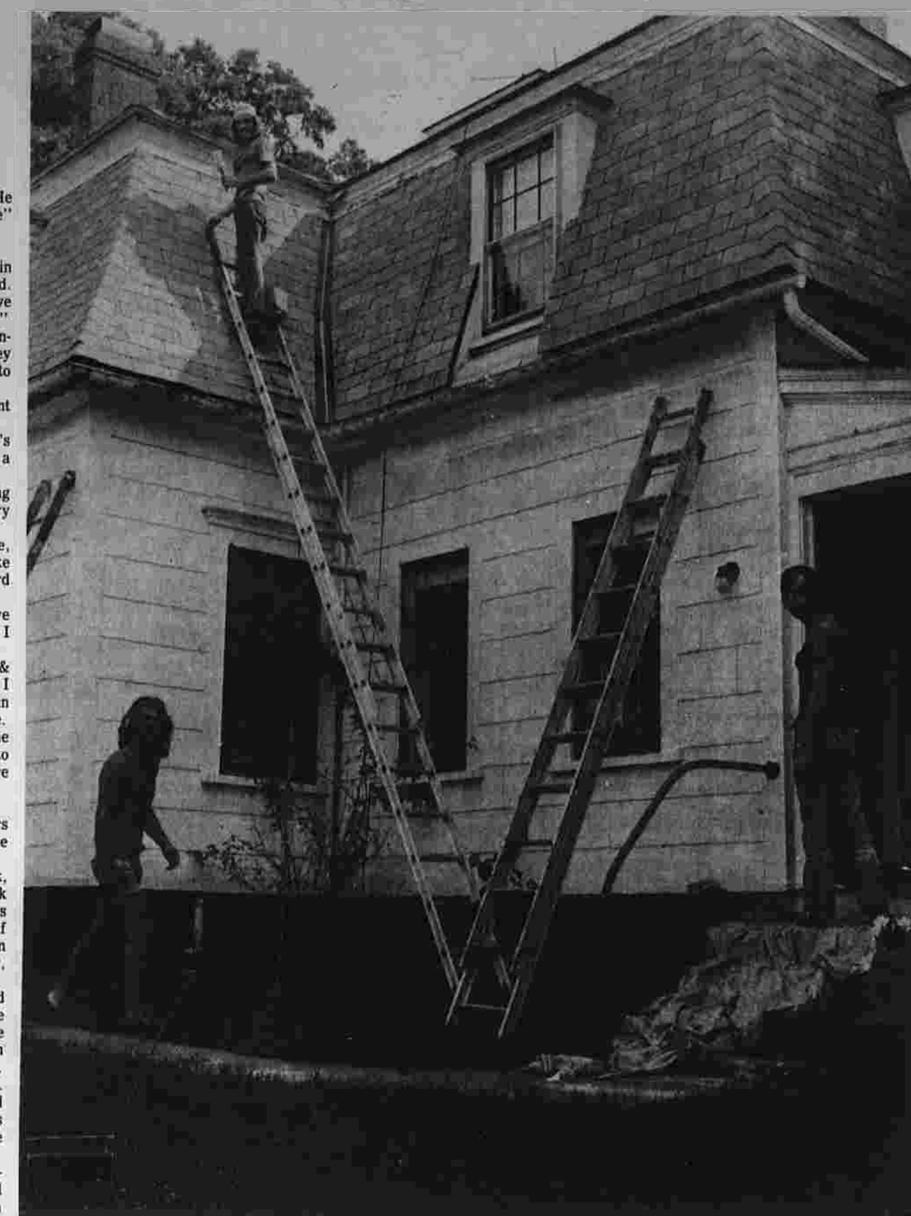
Some of the company are busy painting an older home on Cooper Hill St. They are, from left, Peter Belliveau, Jim Budge, and Mark "Kelly" Palmer. Note the portable radio in the grass. They like to work by music.
